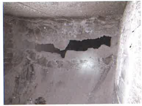
Fig. 2 Refractory damage from alkalis in a kiln with RDF alternative fuel
